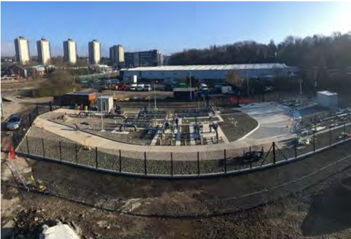
Figure 2.6 Above ground installation example (2)
